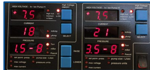
Figure 18: Control Panel of Ion Pumps
